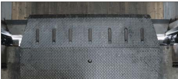
Air gaps at the corners of dock levelers are the source of significant heating and cooling energy loss at many docks.
