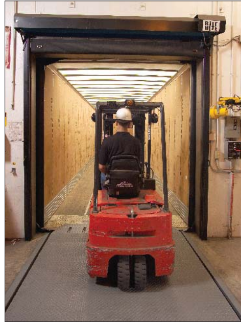
Sealing trailer door hinge gaps with GapMaster hooks prevents energy loss, saving $200 - $1000 per year at each dock position.
