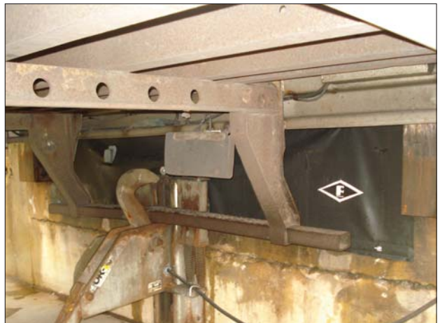
The PitMaster Under-leveler seal is designed to stay in place against the leveler and pit sides during trailer loading and unloading.
